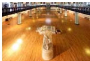
Work begins on the Museum main hall, empty apart from Sir Francis Chantrey's 1830 sculpture of James Watt
