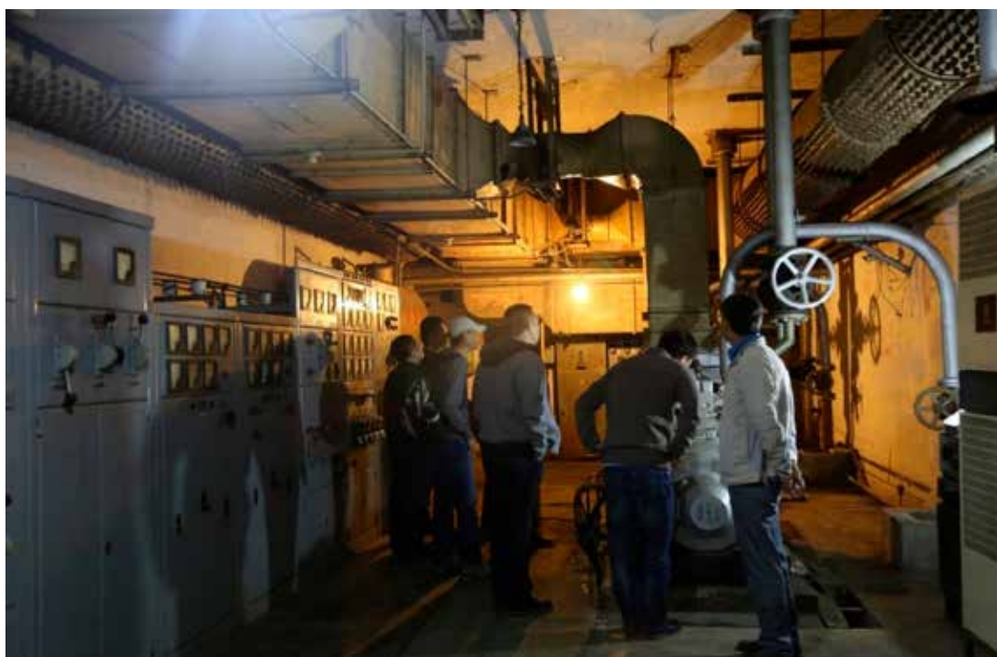
Fig.3 Investigation site of Sichuan International Radio Communication Base (a 10m underground base) Image: Zhao Ke
